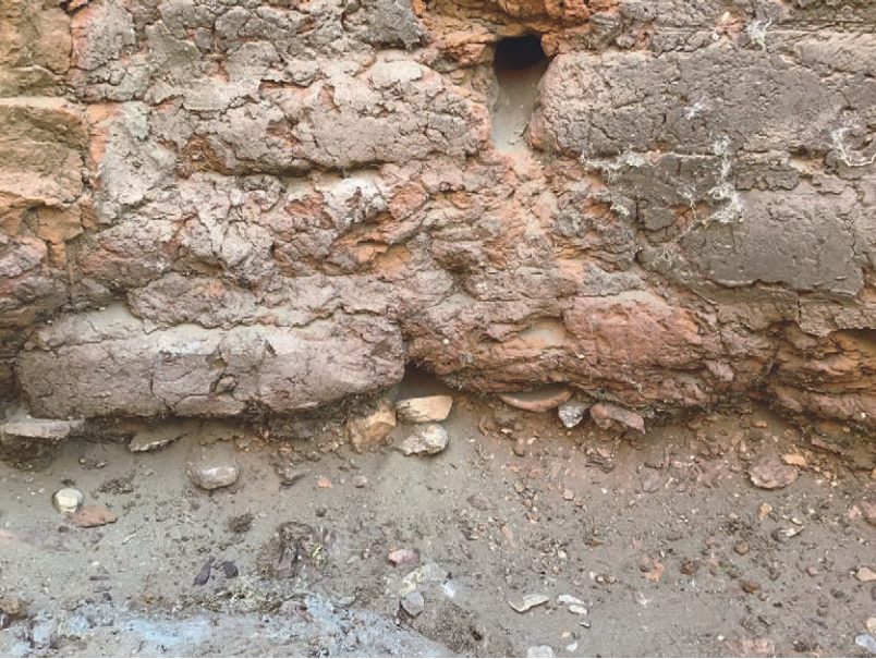
Fig. 8. Details of the lowest course of brickwork and underlying levelling layers containing cultural materials. Photo: URAP; image: C. Knoblauch.
