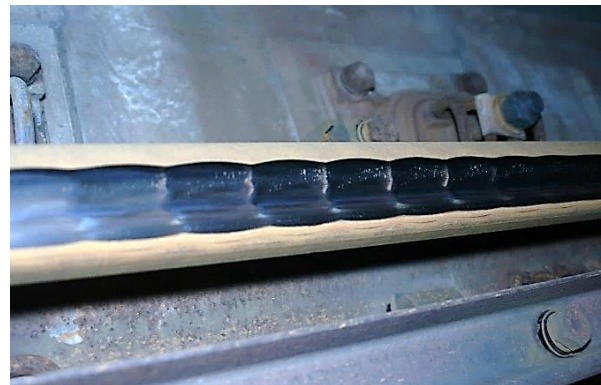
(b) Field rail corrugation condition
