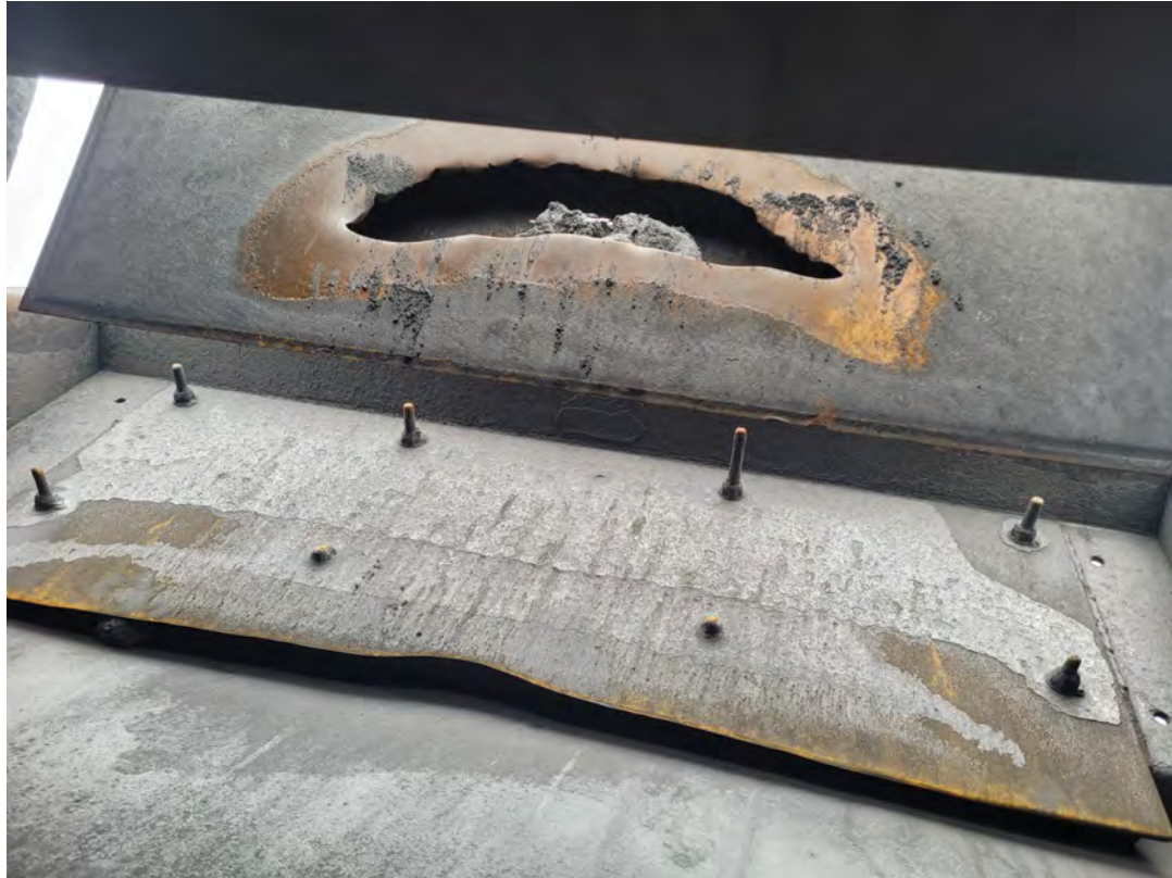
FIGURE 6.11: Coke Screener plate failure after 23 weeks of service
