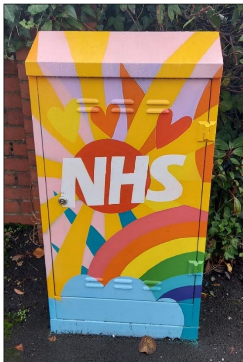
Figure 13: A broadband cabinet in Pontarddulais with a painting on
