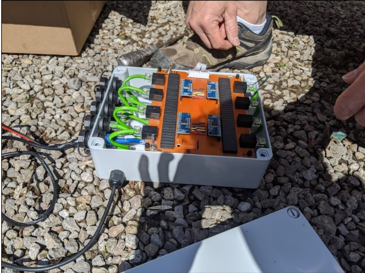
Figure 4.1: Photograph of inside the SPiVolt Hub.
