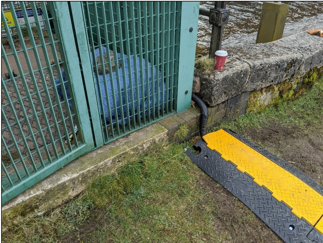
Figure 4.7: Photograph showing SPiVolt cables feeding through speed bump and plastic tubing into valve cage.
