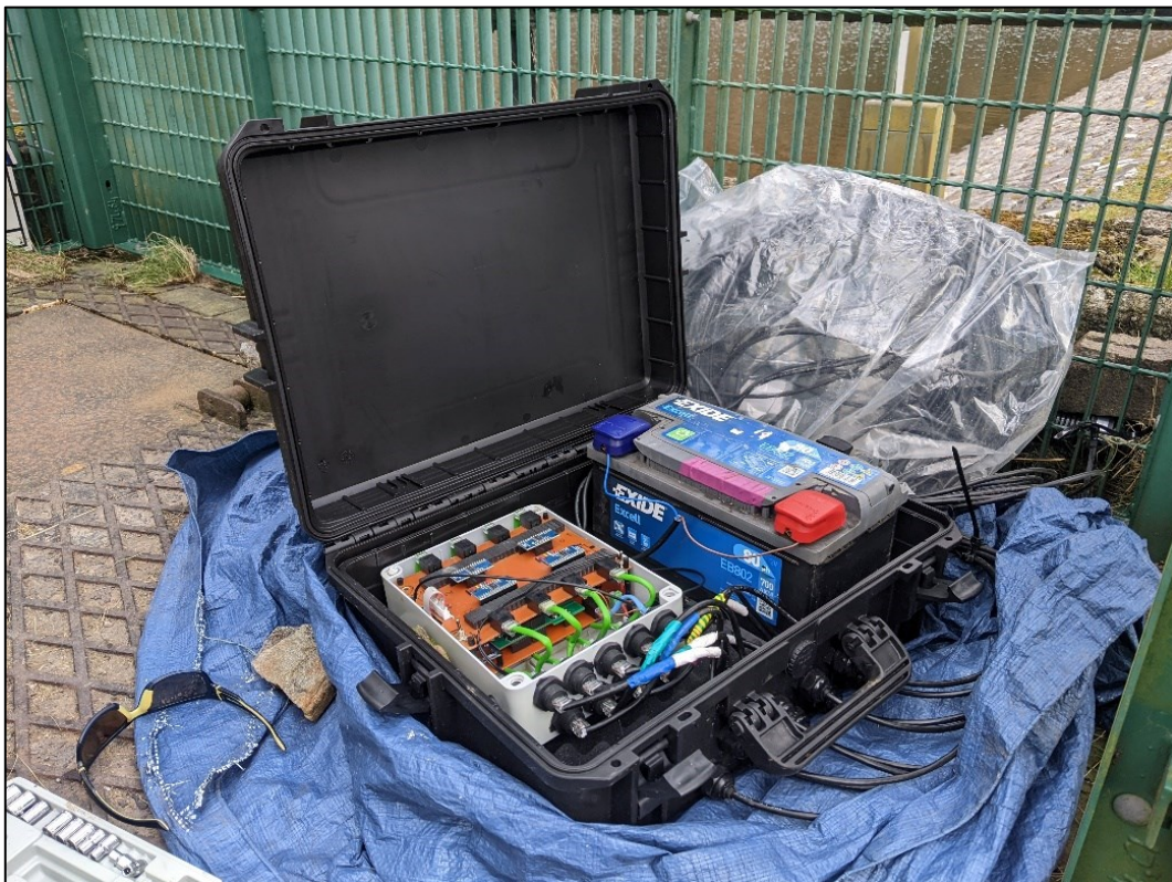
Figure 4.8: Photograph of SPiVolt Hub, power supply and cables secure in weatherproof case with valve cage.
