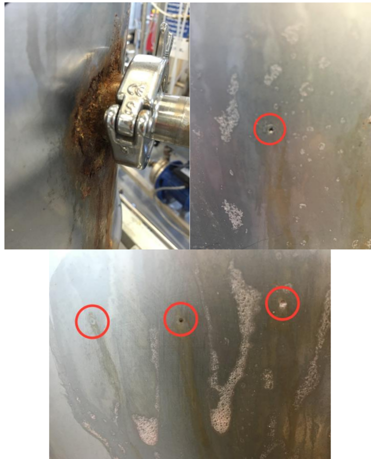
Figure 9. Swanssea feed tank corrosion. Top left, rusting around the tri-clamp connection. Top right and bottom, pitting on the vessel surface.
