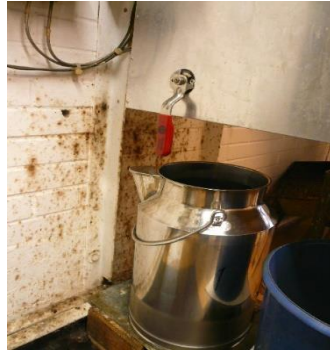
(e) Drain valve (i.e. sampling point)
