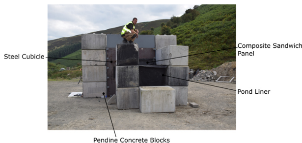
Fig. 2. Photograph showing cubicle and pendine concrete block setup for underwater experiment whilst under construction.
