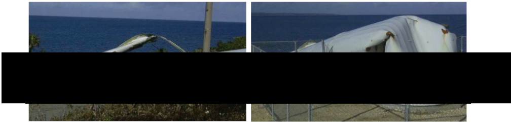
Figure 9.3: Damage to wind energy facilities in Miyakojima island due to Typhoon Maemi, 2003 [114]
