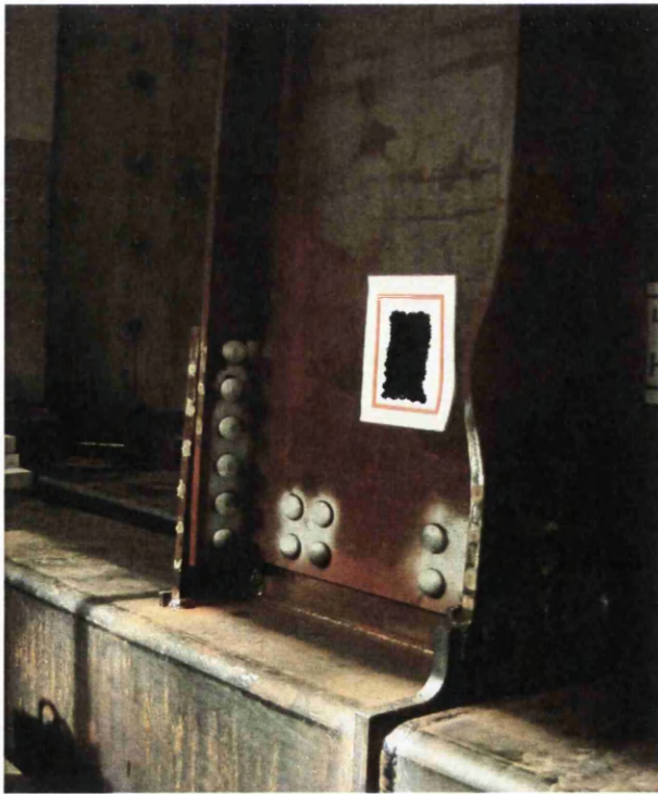
Figure 3.13 Local buckling observed in T-4
