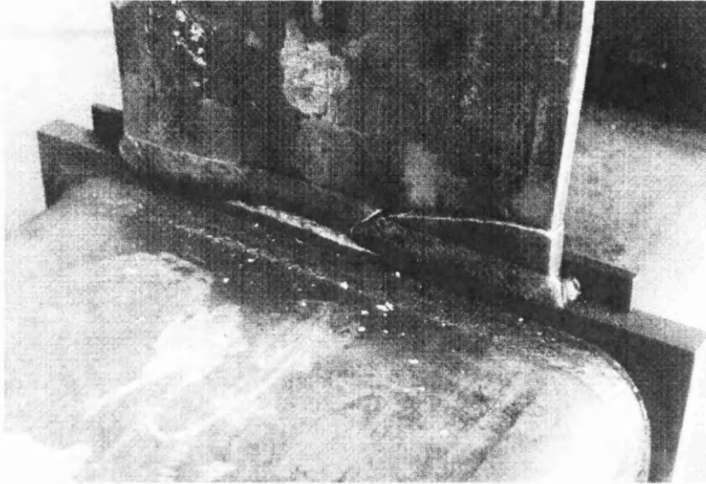
Figure 2.7 Failure mode of conventional connection [Kurobane 1998]
