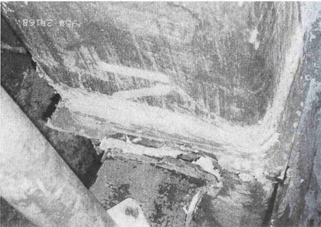
Figure 2.4 Crack begun at weld toe ran through diaphragm [Inoue 1995]
