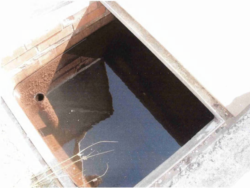
Picture 13: The third of the three interconnected settlement cells, showing the outflow pipe
