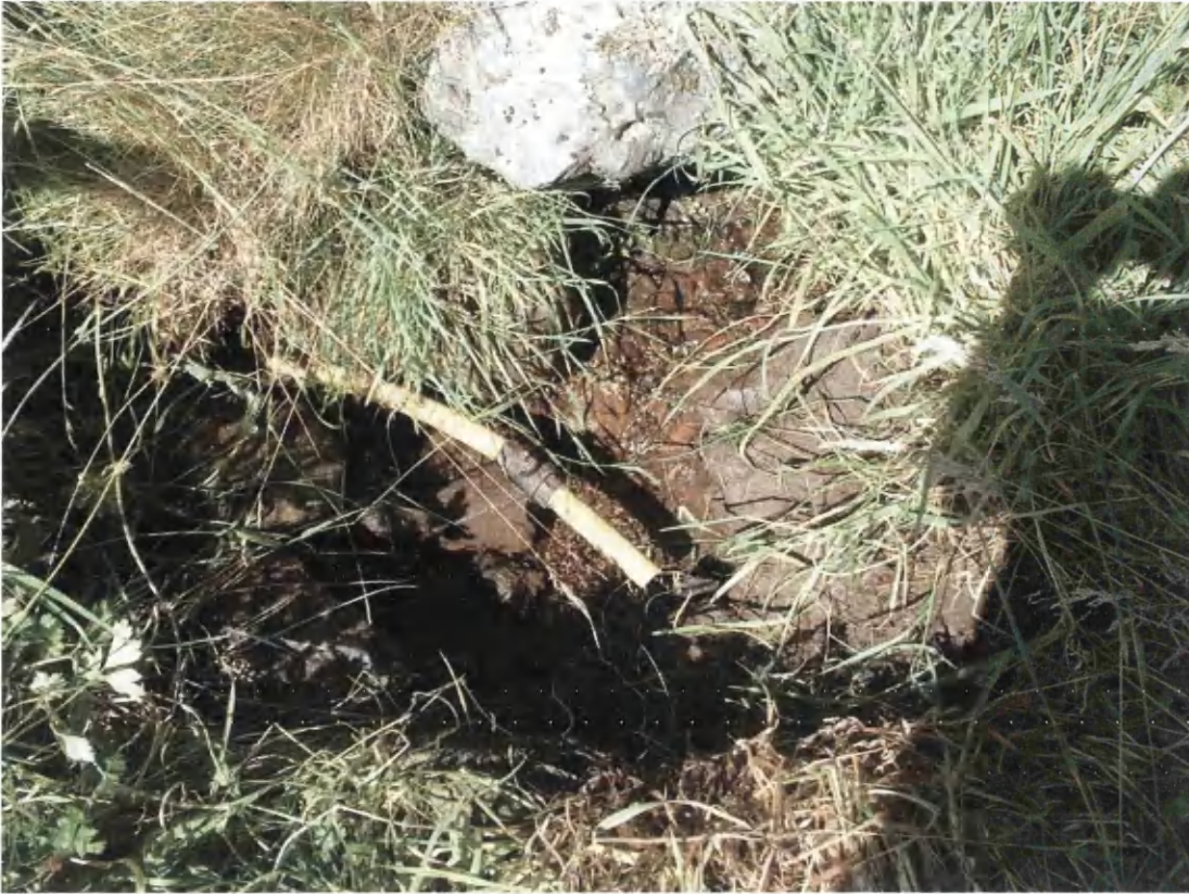
Picture 20: The abstraction point with the corrugated sheet removed, revealing a yellow polyethylene pipe and a small burn
