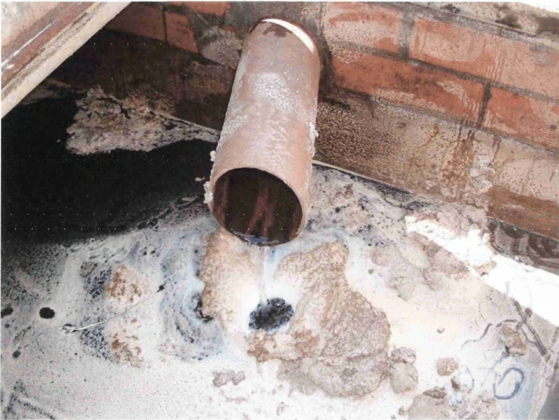
Picture 12: The first of the 3 interconnected settlement cells, showing water flowing from the inlet pipe
