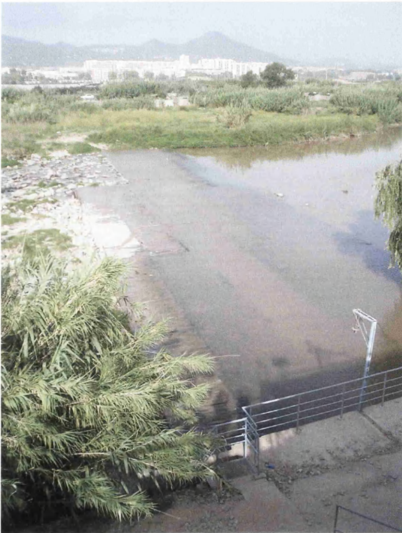
Picture 7: The off-take for the water treatment works
