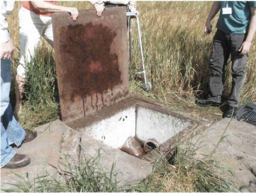
Picture 17: One of the metal sheets removed, to reveal the settlement chamber and the inlet pipe (curved downwards) and the outlet pipe (to the right of the inlet pipe)
