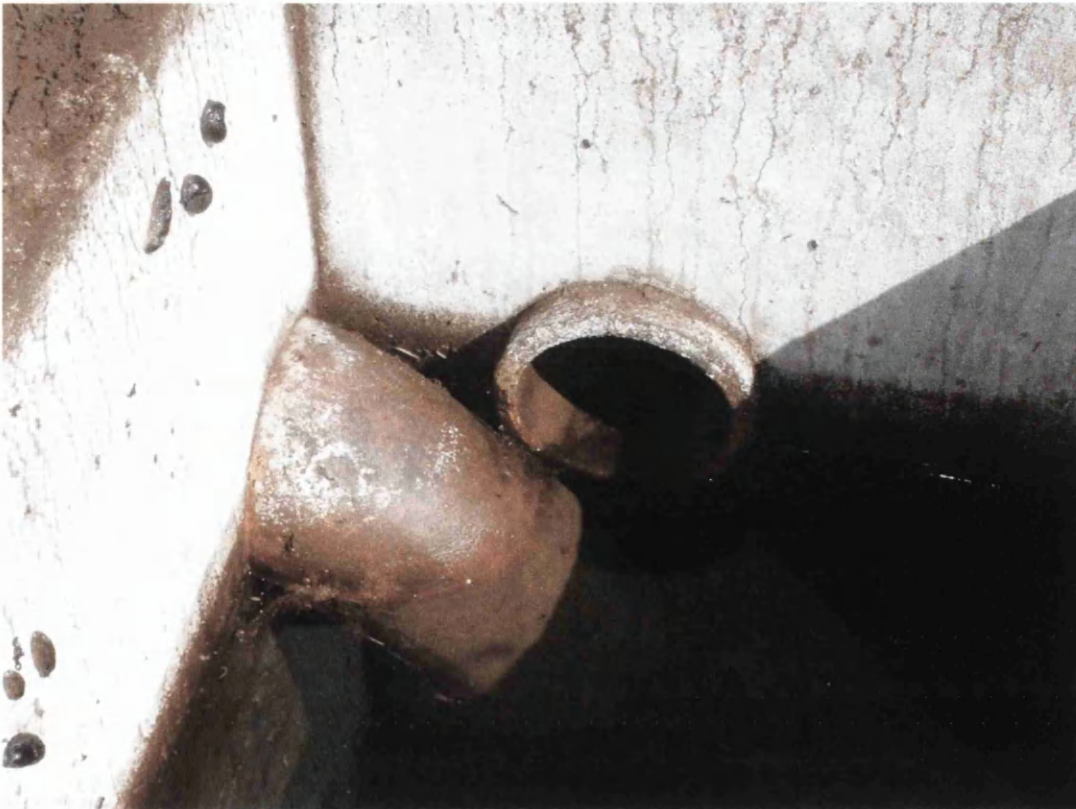
Picture 18: Close-up of the inlet and outlet pipes
