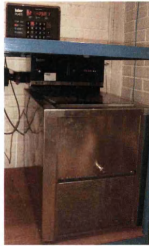
(b) Refrigeration system
