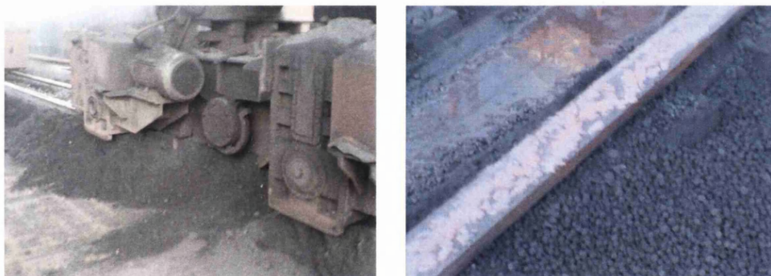
Figure 169: Material spillage encroaching onto crane bogies and rails
