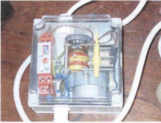
Figure 87 Electronic timer constructed to produce one 12s on-phase per hour.
