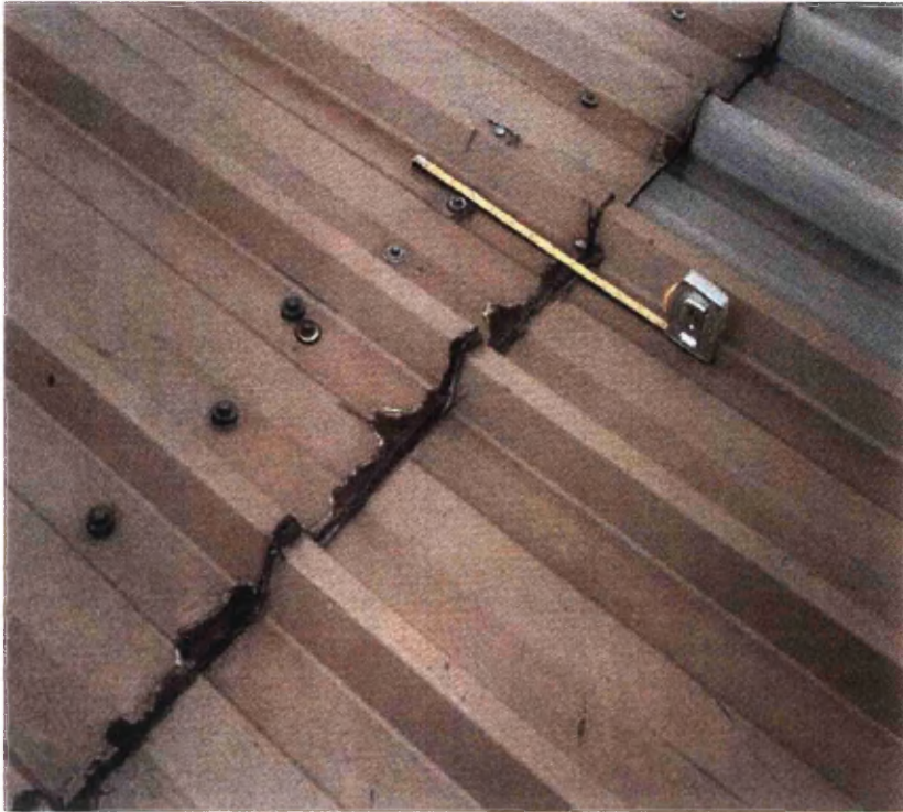
Figure 1.4: The corrosion of the metal substrate at a cut edge.
