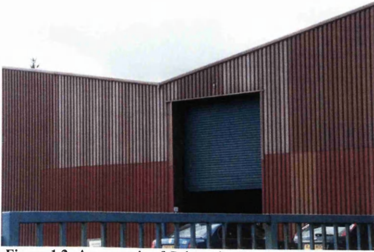
Figure 1.2: An example of Colour change and fading making the building unsightly and any replacement panels obvious.
