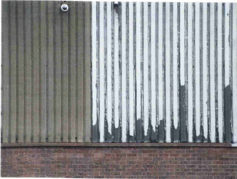
Figure 1.3: Faded Van Dyke Brown OCS same original dark brown colour different supply origin showing delamination and exposure of galvanized substance on the right (grey colour).
