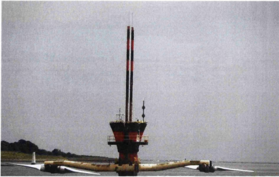
Figure 1.1: The SeaGen turbine installed in Northern Ireland. Image Copyright Kenneth Allen. This work is licensed under the Creative Commons Attribution-Share Alike 2.0 Generic License.
