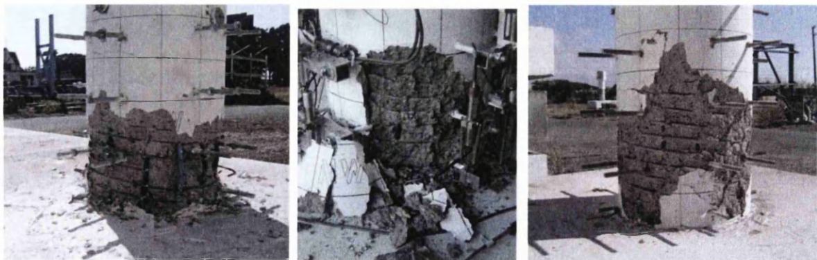
Figure 2.14 Damages in specimens at plastic hinge zones [51]
