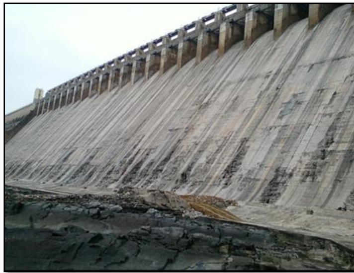
Figure 1.14 Cavitation damage on spillway profile of Nagarjunasagar Dam ( https://www.ecronicon.com/ecag/agriculture-ECAG-01-00004.php ).
