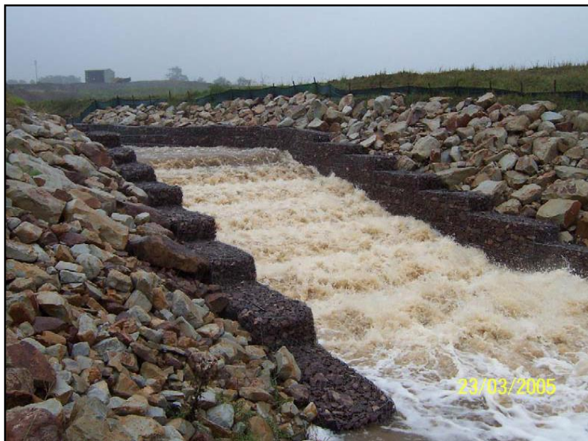
(a) Diversion stepped channel at Duralie Coal project (Australia) on 23 March 2005 (Courtesy of Tony Marszalek).
