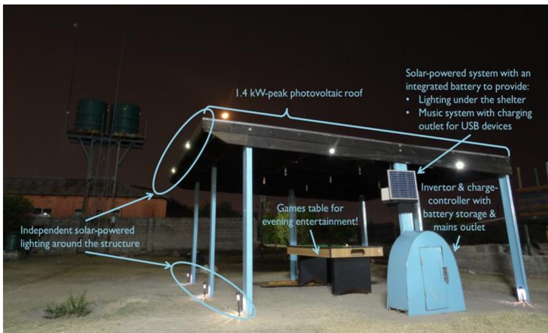
Figure 7.2 Off-grid solar energy structure with 1.4 kWp of integrated PV in an orphanage in Mutende, Lulamba, Zambia
