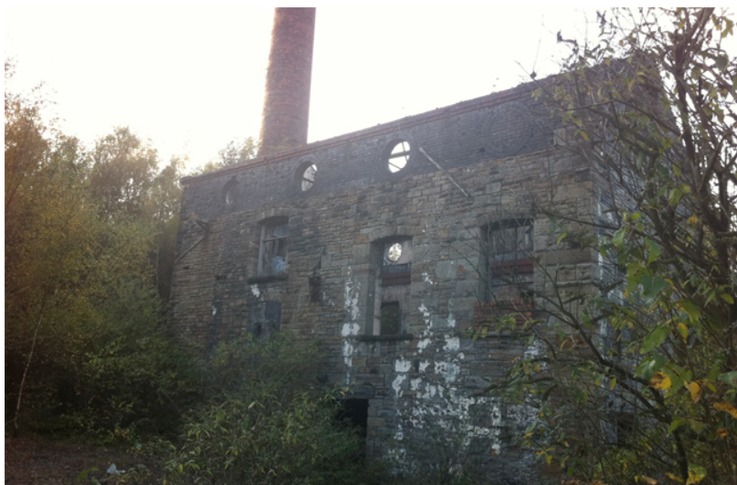
Fig. 1 A crumbling building at the Hafod Copperworks (2012)
